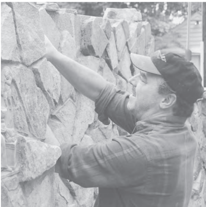
Stonemasons often work from a set of drawings in which each stone has been numbered for identification
