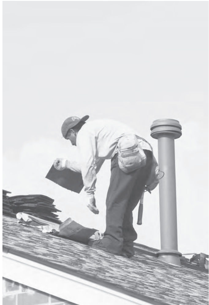
Starting from the bottom edge, roofers staple or nail overlapping rows of shingles to the roof.
