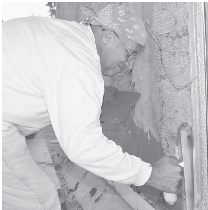
Plastering—one of the oldest crafts in the building trades—remains popular due to the relatively low cost of the material and its overall durability.
