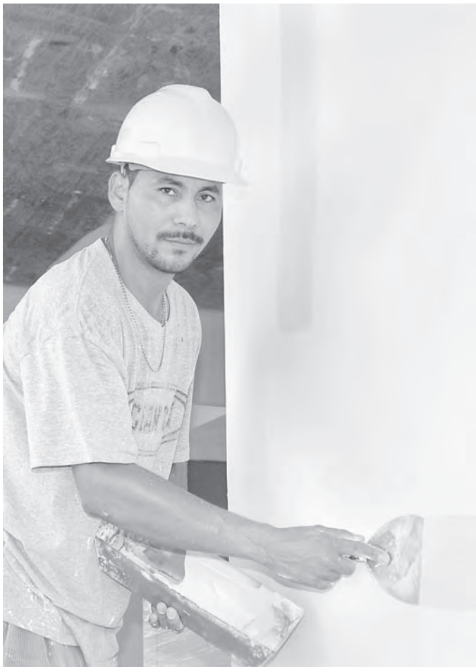
After the drywall is installed, tapers fill joints between panels with a joint compound.
