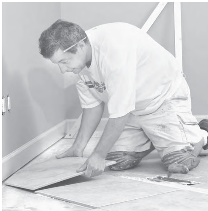
In order to cover all exposed areas, including in corners and around pipes, tilesetters use a machine saw or a special cutting tool to cut tiles to fit.
