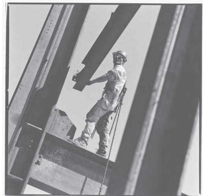
Because the danger of falls is great, ironworkers use safety devices such as safety belts, scaffolding, and nets to reduce risk.
