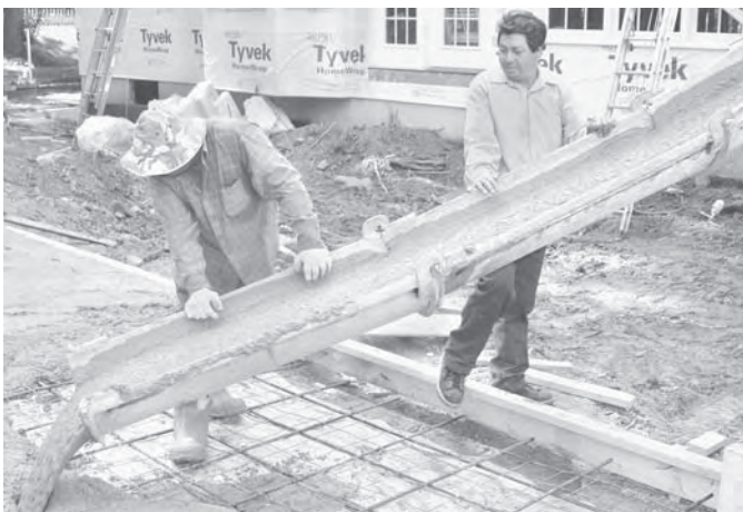
Cement masons and concrete finishers spread the concrete, and then smooth and finish the surfaces.
