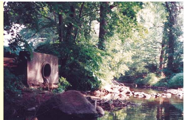
Figure 9. Unregulated impervious-area runoff directly affects water quality, habitat, and aquatic communities in streams and is exemplified by a storm-sewer pipe (left) that drains directly into the Saddle River at Ridgewood, N.J.
