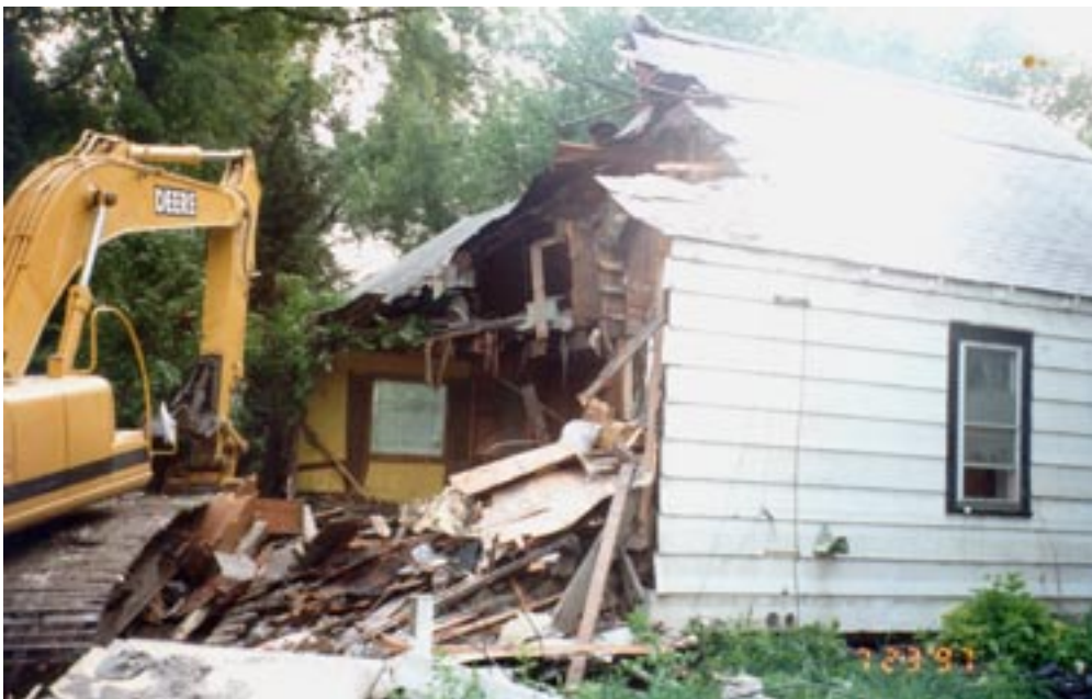
Demolition was the best option for the Arntz's flood-ravaged home. The couple was the first to voluntarily sell their home to the city. Under the terms of the buyout, the land will forever remain as open space. Photo courtesy of Cliff and Eleanora Arntz.
