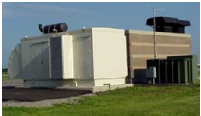
A backup generator enables this lift station (brick building) to operate during a power outage.
