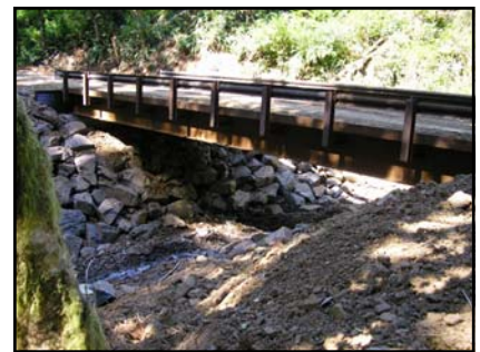
The Roscoe Steel Bridge was installed over an unnamed tributary to East Humbug Creek during the summer of 2005.
