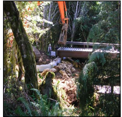
A bridge is constructed over a tributary of the East Fork Humbug Creek.
