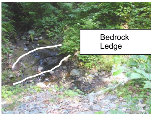
Figure 6. Upstream of the culvert, the channel has exposed a bedrock ledge that is a low flow passage barrier.
