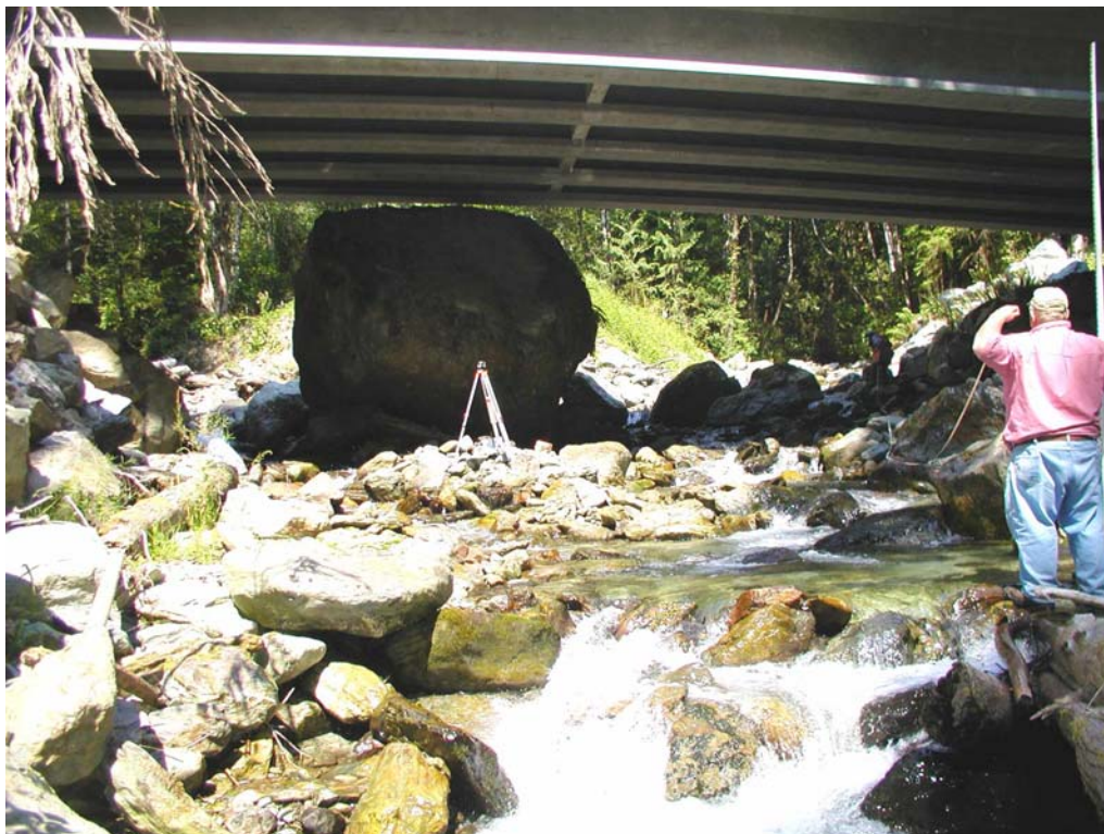
Figure 13. Road 1100000, MP 23.7. Bridge replaces two culverts that were located in each channel where there is sunlight in the photo. Channel gradient under the bridge is 7 percent; the left channel upstream is 20 % gradient; the right channel is 11 %. The large center boulder sits under the bridge.
