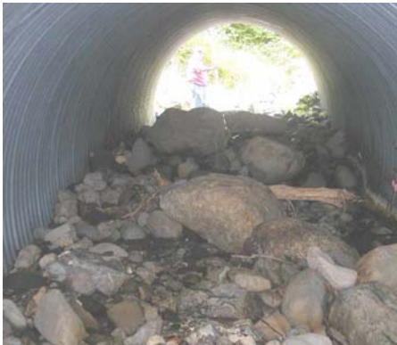
Figure 9. Substrate scour within the pipe. Fluorescent orange paint marks level of substrate when installed. Depth of scour on right is 2.5 feet.
