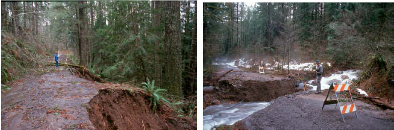
Figure III-11 - Examples of Catastrophic Fill and Culvert Failure from the Mt. Hood National Forest Roads Analysis (examples are not in the Bull Run Watershed Management Unit)
