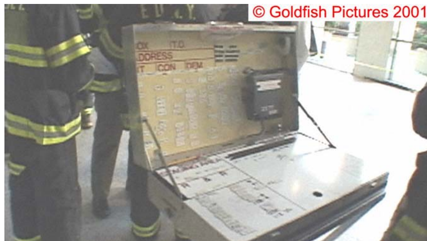
Figure 7–7. Fire Command Board located in the lobby of WTC 1.
