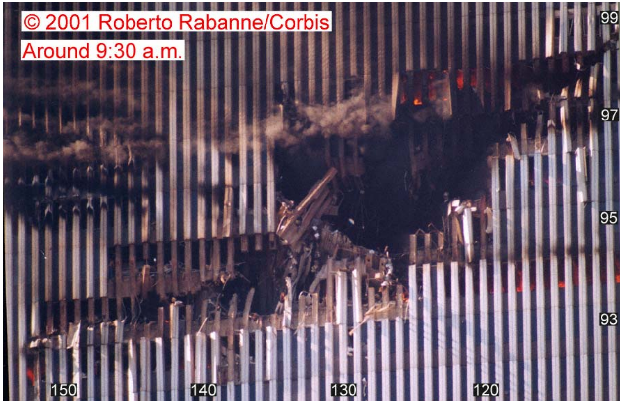
(a) Observed Damage
