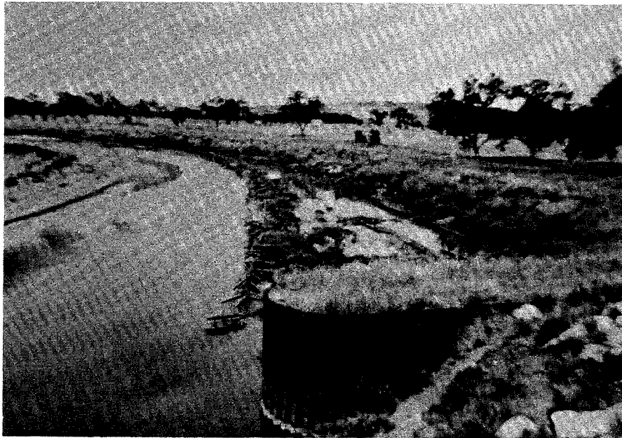
Figure 15. Steel sheet-pile spur (wing dam) upstream from bridge. Kellner jack field along bankline beyond spur. (Grand River, S. Dak., Site 175; photograph from South Dakota Dept. of Transportation.)
