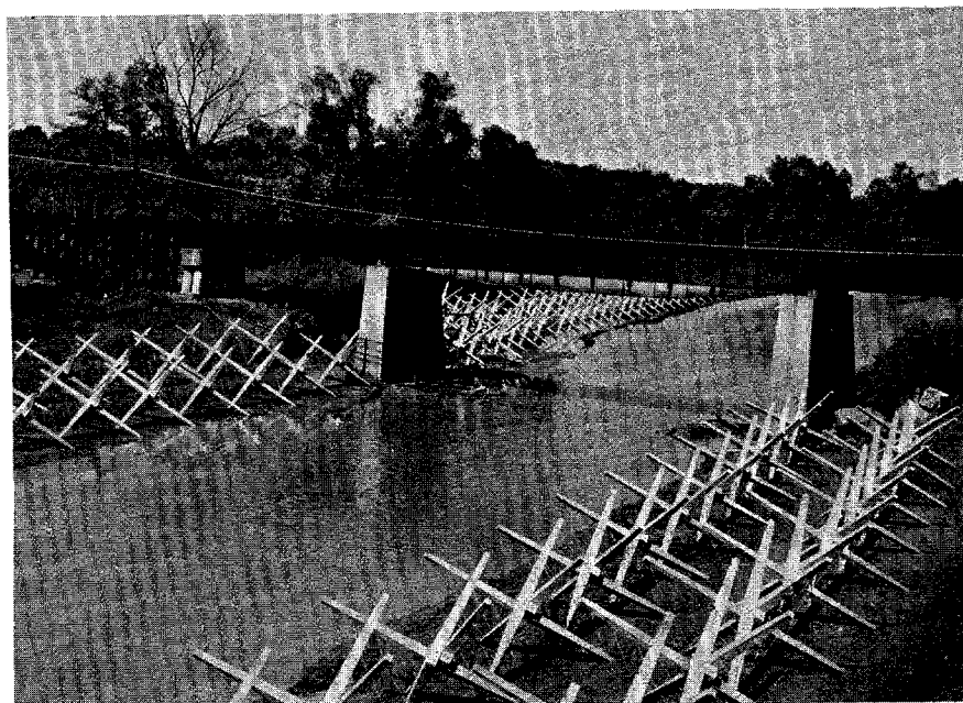
Figure 21. Concrete jacks used as retards, photographed soon after installation in 1970. (Tallahatchie River at New Albany, Miss.; U.S. Dept. of Agriculture, Soil Conservation Service.)
