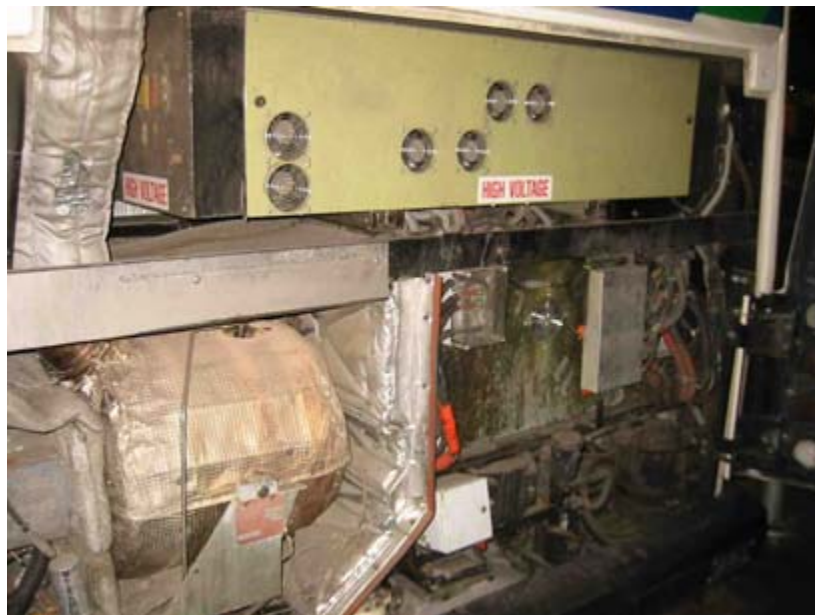
Figure 14. Capstone MicroTurbine Assembly (Source: NREL)
