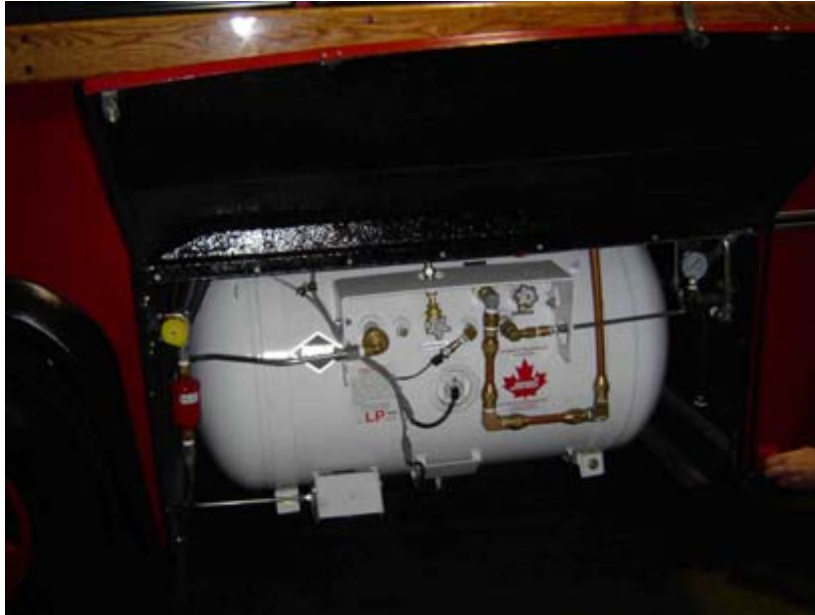
Figure 22. On-board LPG storage
