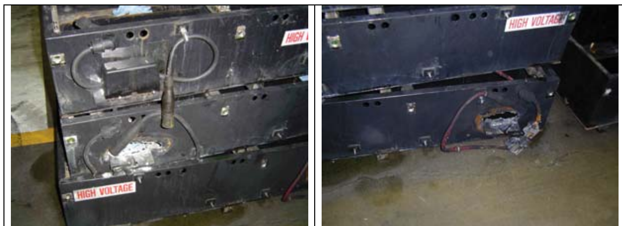
Figure 6. Normal battery tray (left) and tray with a corroded cable (Source: NREL)
