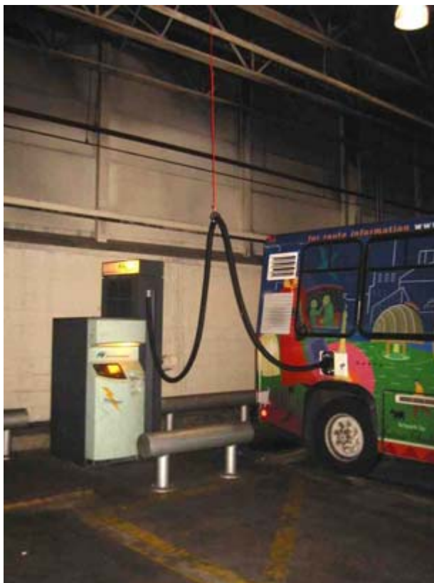
Figure 15. IndyGo Ebus at Charging Station (Source: NREL)
