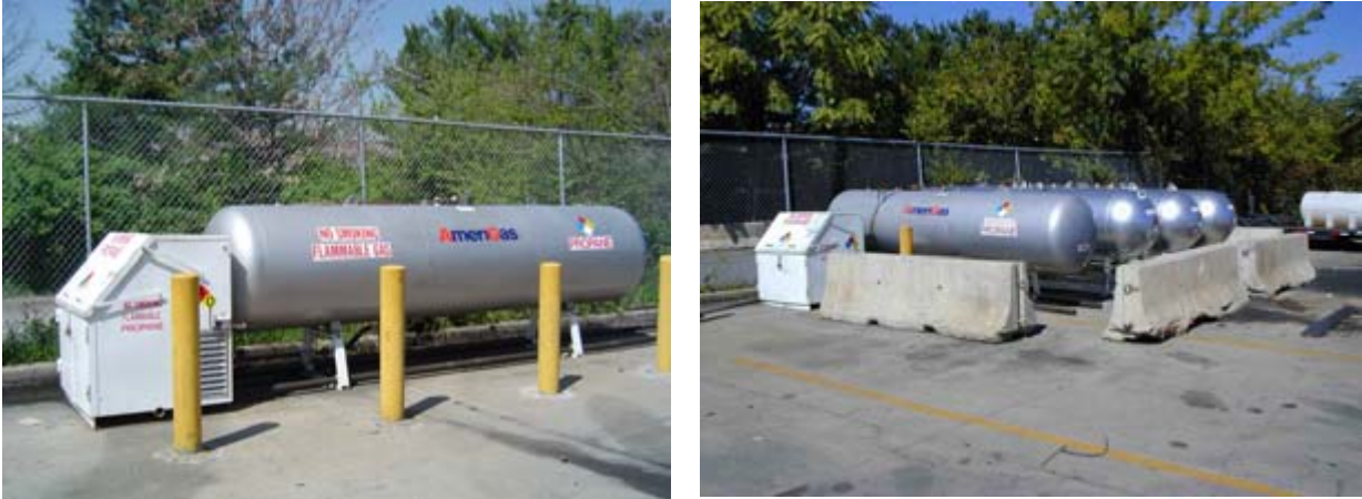
Figure 21. Original and upgraded LPG fueling station
