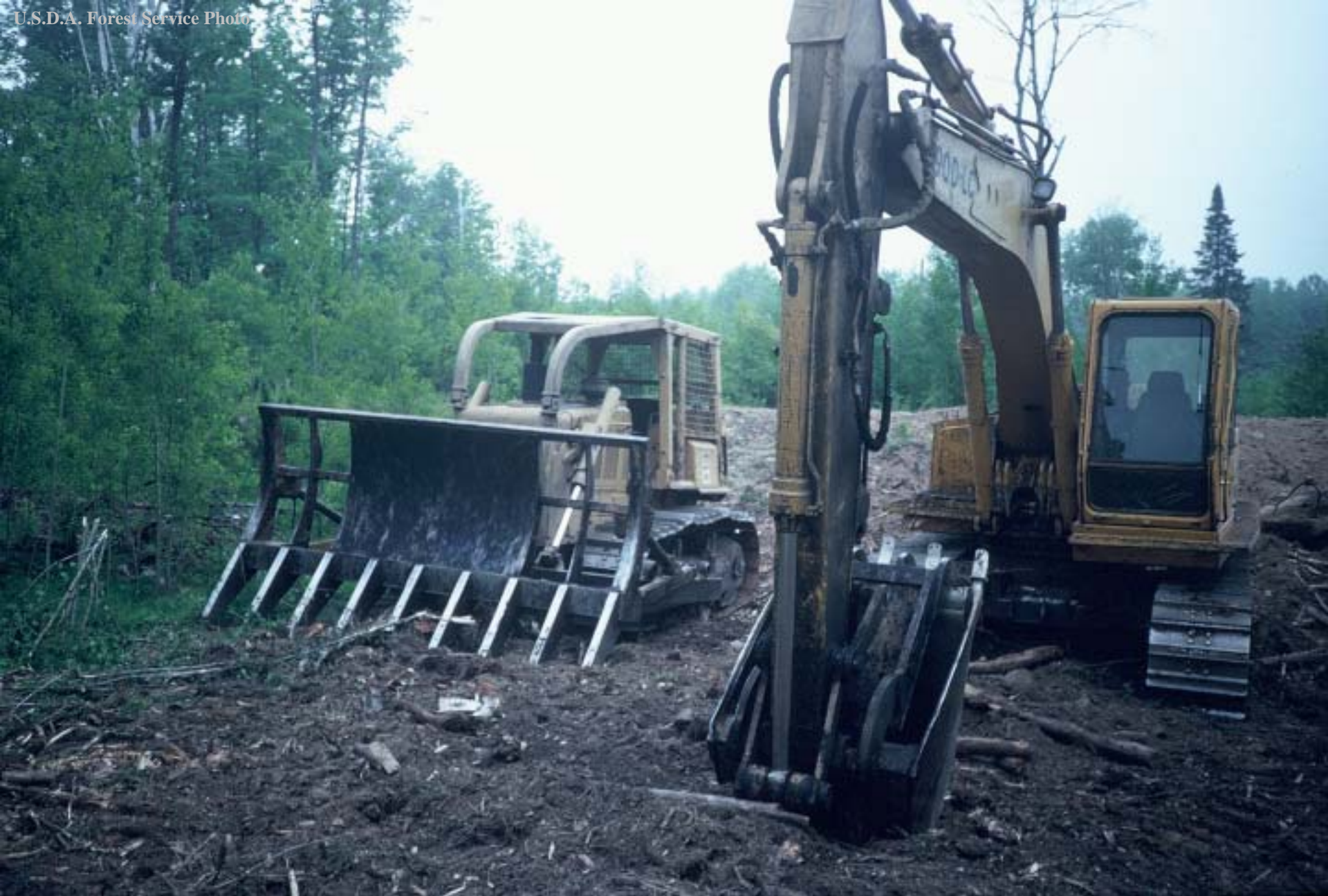
Equipment at Pipeline Location
