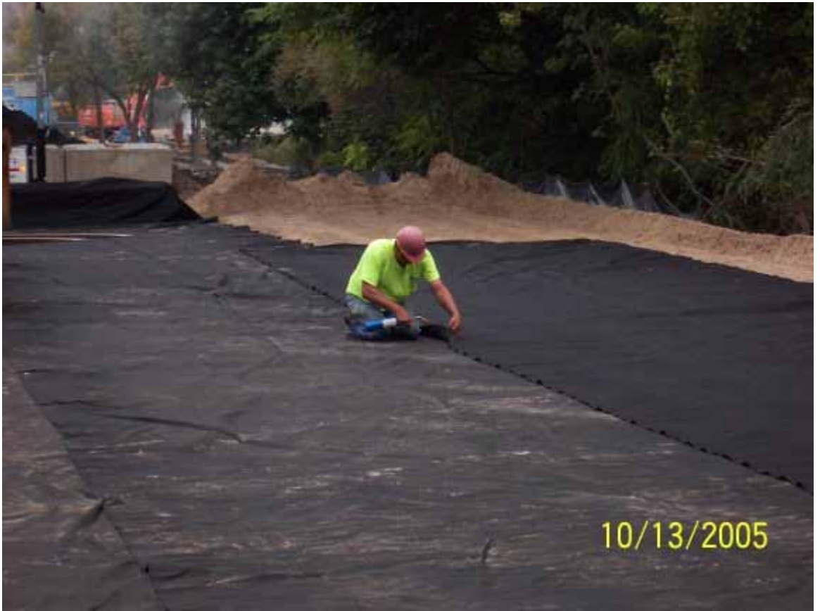
A worker takes great care to heat-seal membrane joints by warming the fabric with a torch.
