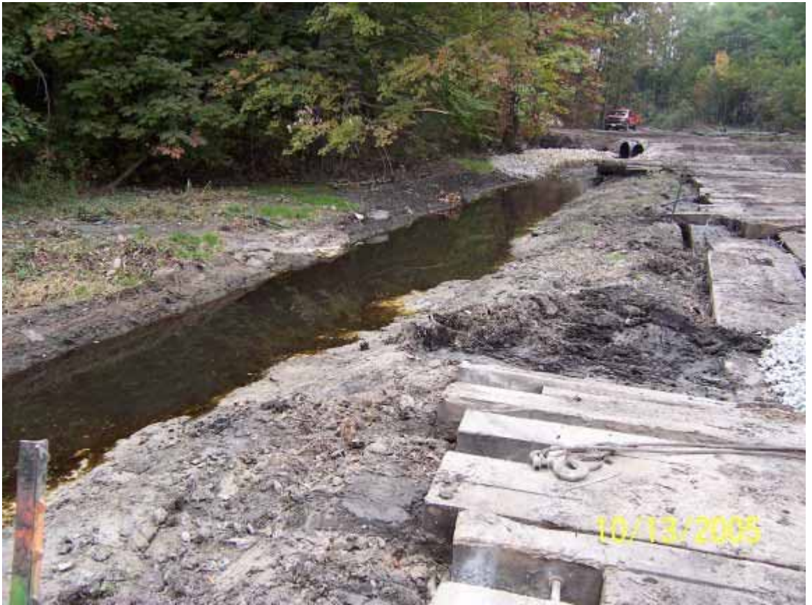
Here is the new creek channel viewed downstream of the diversion culvert. Note the timbers of the haul road on the right side.
