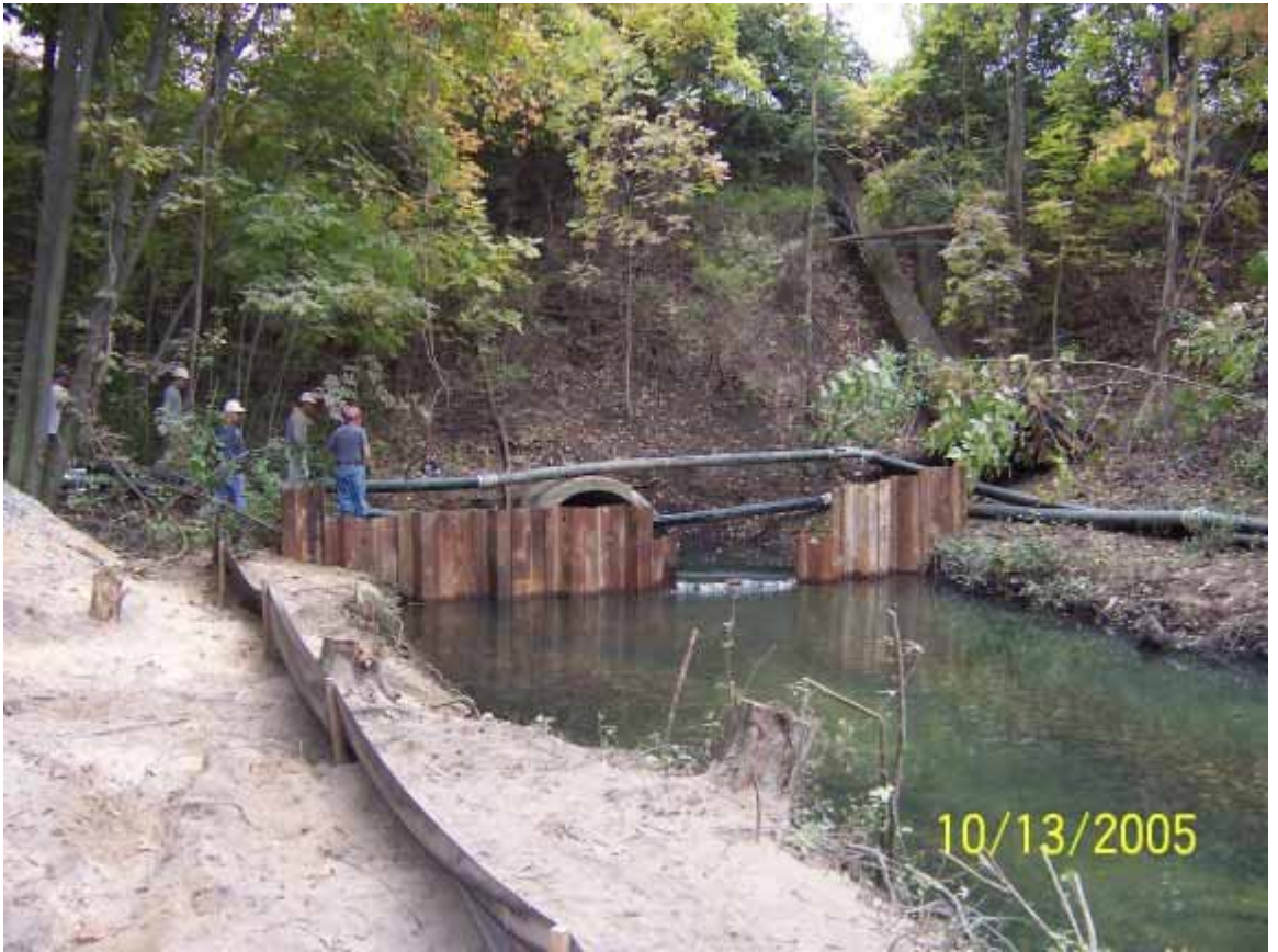
Here Jackson-Merkey workers are preparing this reach of the creek for sediment excavation.
