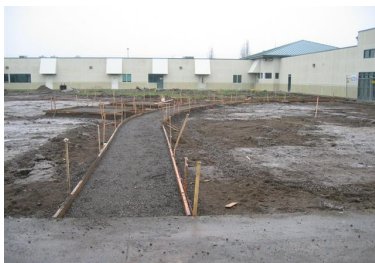
(Above) Significant ground transformation is taking place in the courtyard to create the pathways and picnic table areas.
