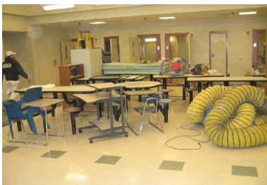
(Above) The contractor staged tools and materials in the living units to facilitate efficient execution of the work.
