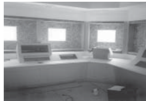
Central Control Room
