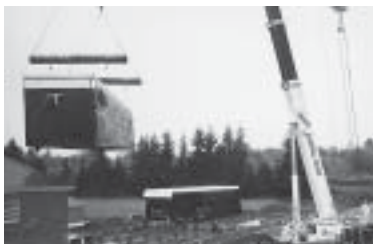
Cranes were used to lift and place the pre-fabricated modular structures among the long-standing brick buildings of Hillcrest.
