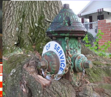
An out of service fire hydrant in DC Credit: Dave Statter, WUSA9 News
