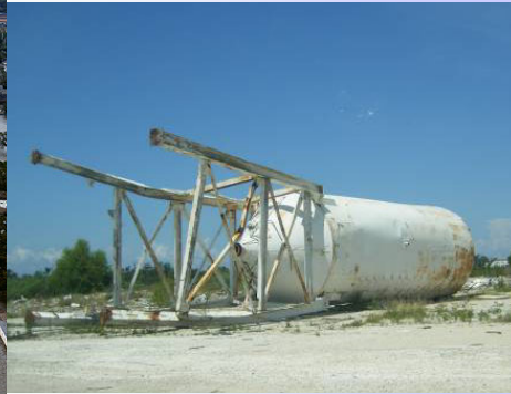
Fallen water tower in Biloxi, Mississippi caused by Hurricane Katrina, August 2005
