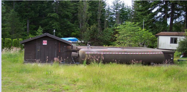
Small system wellhead with hydrotank
