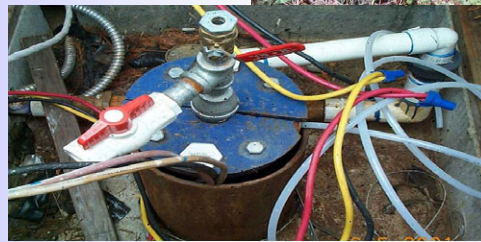
Wellhead that needs to be replaced
