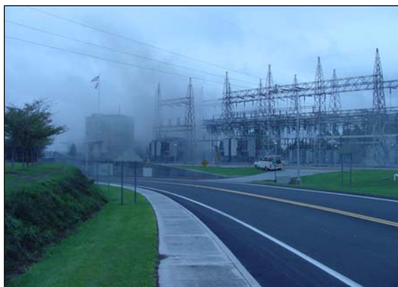
Control building and switchyard, looking southeast on Highway 68
