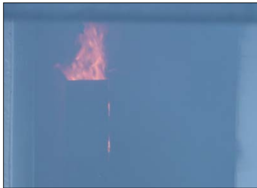
Fire in the breaker panels; looking from outside the Control Building, three hours into the fire.
