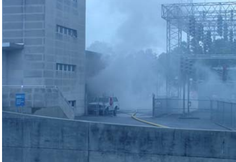
Control Building, approximately two hours into the fire
