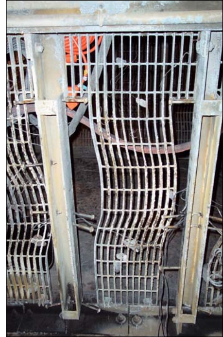
Warped decking below the area of origin
