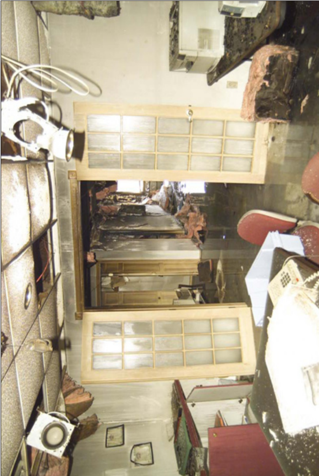
9. The Barn's second floor, looking south from the conference room. This room sustained only heat and water damage due to the presence of a wood floor in the attic. Office G can be seen through the French doors. It was devastated.
