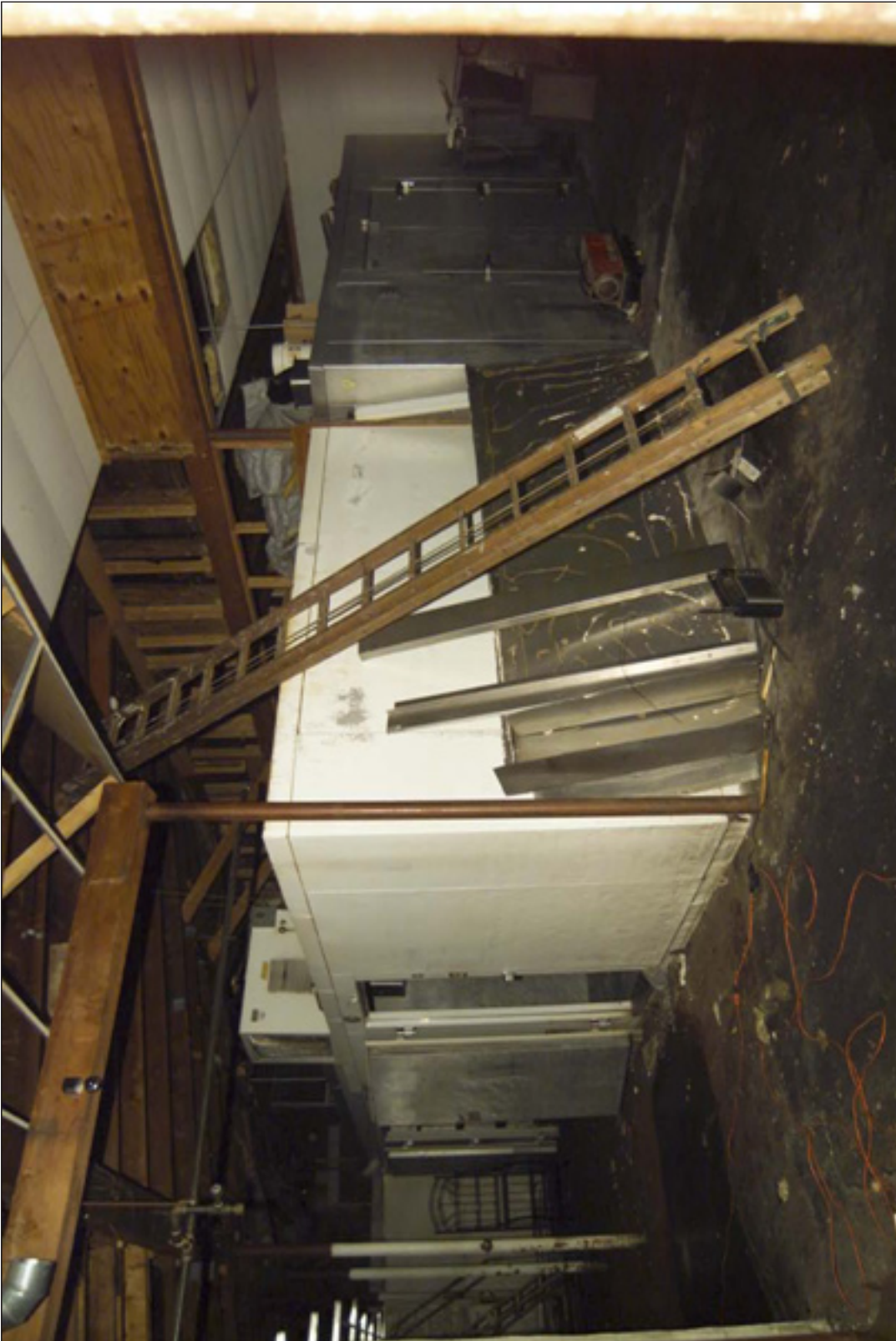
10. These are the walk-in coolers at the east end of the complex. The smoke damage was minimal, and $40,000 worth of inventory was saved.
