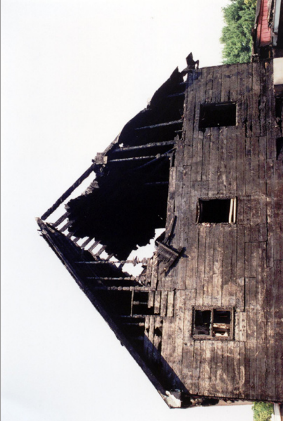
3. The upper part of the Barn's C side. The gable had burned through before firefighters arrived. The unstable roof was removed after suppression was completed.
