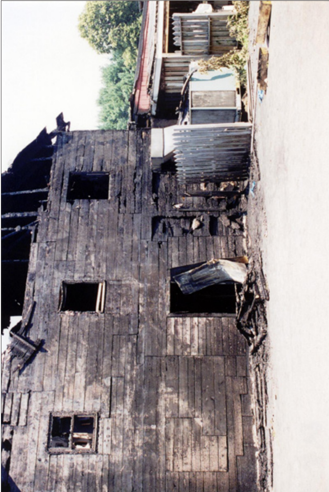
4. The lower portion of the Barn's C side. This surface, finished with vinyl siding, was engulfed when firefighters arrived. The area of origin is at the lower right.
