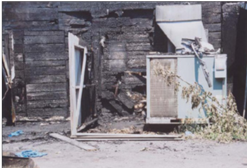
The area of origin viewed from the south on the morning of the fire. Note the penetrated sheathing and protruding wires from the electrical service.
