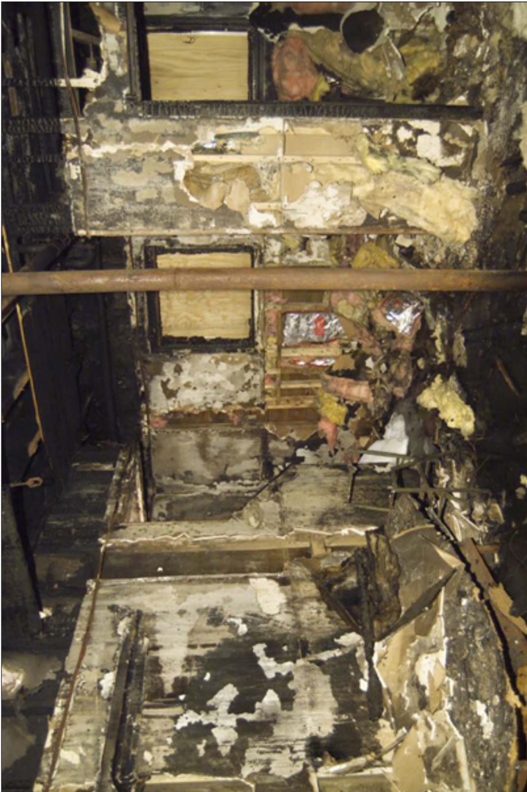
8. Another view of the employee area, looking southwest. The entrance to the staircase is at the end of the left wall where it intersects with the west wall, the C/D corner of the Barn. Fire damage in this area was caused by debris dropping down from above. The interior attack extinguished the fire in the room.
