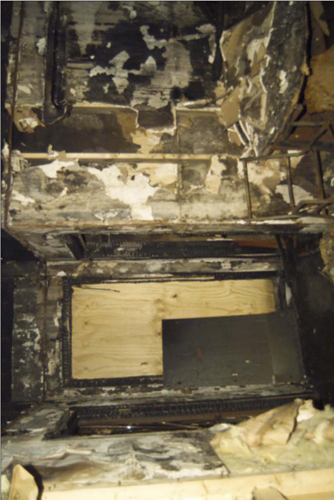
7. The employee area on the Barn's 1st floor, looking south at the D6. The electrical room is through the door on the left, and the door on the right accesses a closet under the rear stairway to the second floor.
