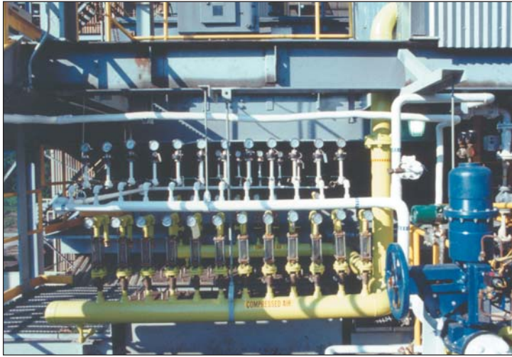
CZD/FGD lime slurry injector control system.
