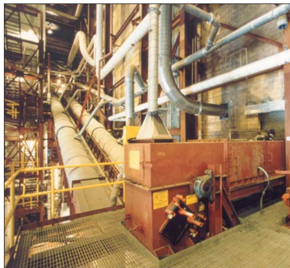
Coal and sorbent conveyors can be seen just after entering the Tidd plant.
