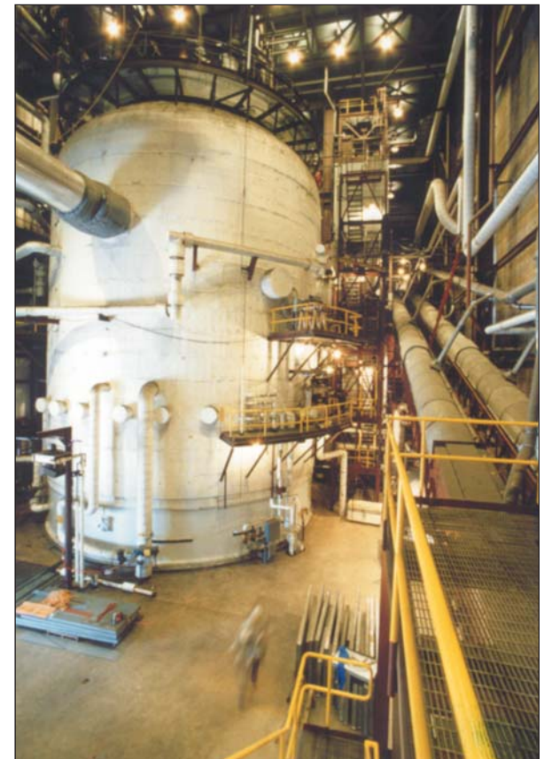
Pressurized fluidized-bed combustion, like that demonstrated at Ohio Power Company's Tidd Plant, is starting to see global commercialization.
