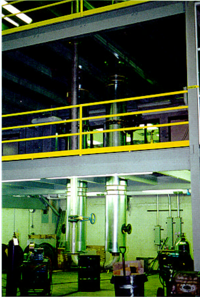
Exhibit 2.2 -24 Photograph Of Installed/Insulated Tube-And-Shell Heat Exchangers
