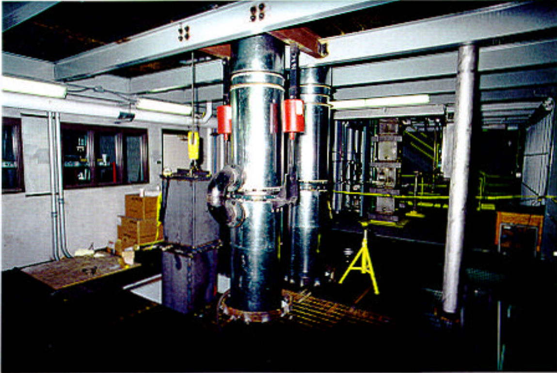
Exhibit 2.2-23 Photograph Showing Cooling Air Preheat Shell Sections Being Installed Adjacent To Tube-And-Shell Heat Exchangers
