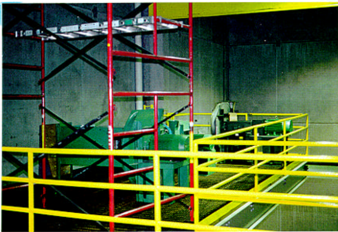
Exhibit 2.2-26 Photographs of system fans
