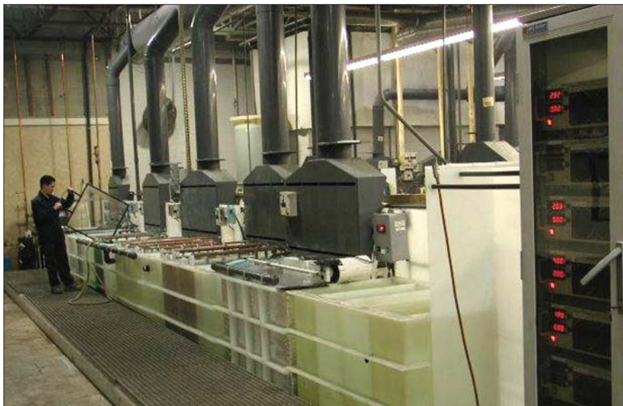
OSHA's hexavalent chromium rule will require new exposure controls from a variety of industries, including electroplating (shown here); welding; aerospace and auto body painting and repair; chromate pigment and chemical production; glass manufacturing; and plastic colorant production.
