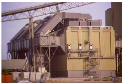
Full Scale Advanced Hybrid™ Retrofit at Big Stone
