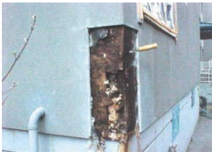
Moisture leakage into this stucco wall system has led to severe rotting of this six-year-old building in Seattle.
