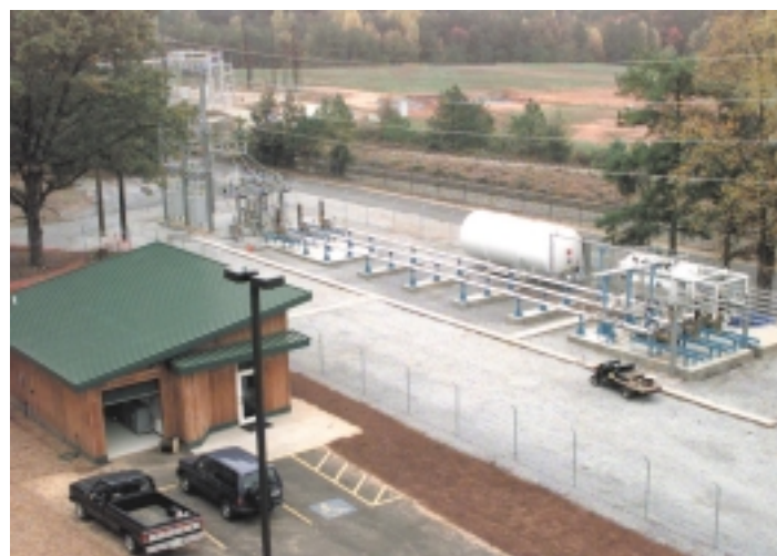
The world's first field test of an HTS power delivery system will deliver power to three plants at the Southwire facilities.
