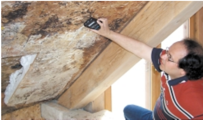
BTC research scientist Achilles Karagiozis measures moisture levels in a roof damaged by moisture intrusion.
