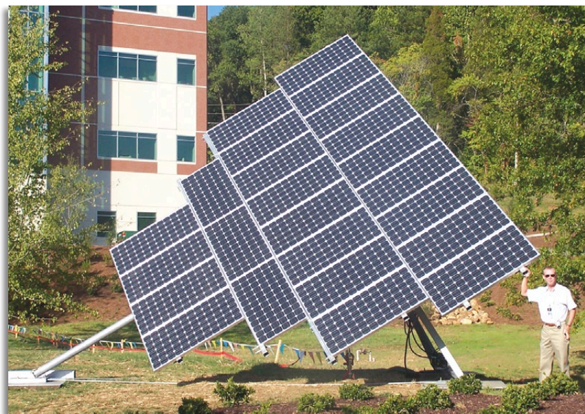
The Arizona Public Services single-axis tracker installed on the ORNL campus was dedicated at the Solar Summit.
