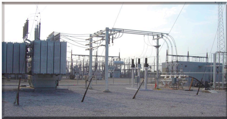
AEP Bixby substation where the Columbus HTS cable is installed. The photo shows the cable emerging from an underground duct, termination, and overhead tie-ins to the AEP grid.
