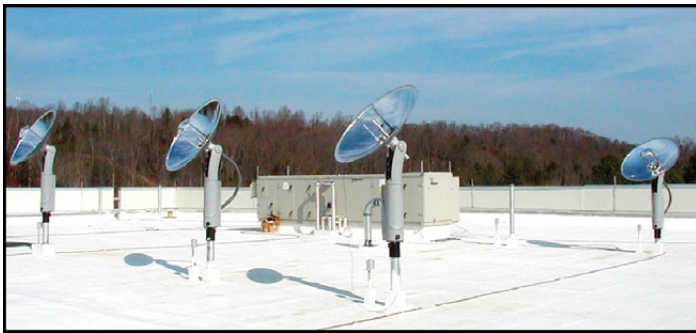
HSL systems atop ORNL's Multiprogram Research Facility.
