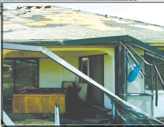
Broken glass in doors (bottom) allowed winds from Hurricane Charley to enter and pressurize the interior of this Florida residence, blowing the plywood roof decking upward and destroying the roof (top).
