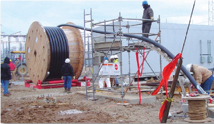
Pulling the vacuum-jacketed flexible cryostat into the underground duct at the Bixby substation.
