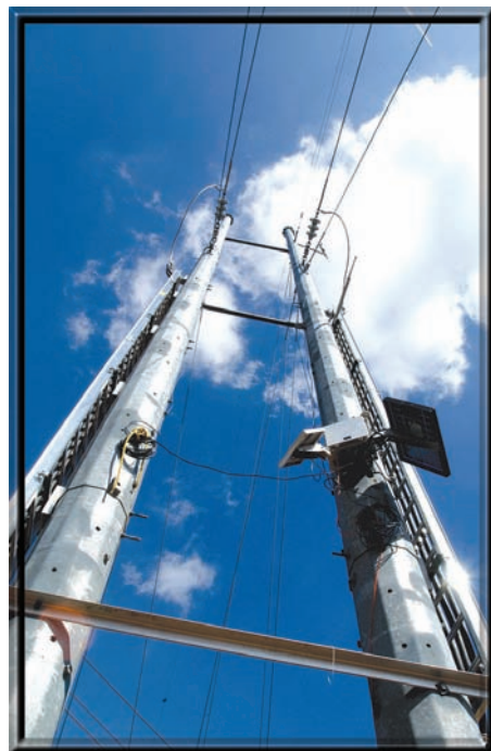
Power cables being tested at ORNL's PCAT facility on Bethel Valley Road.
