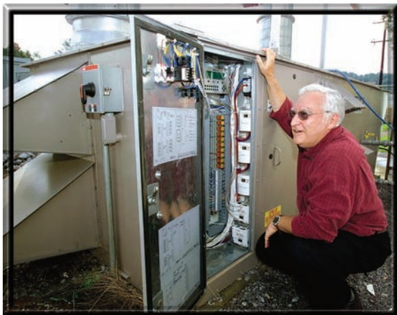
Jim Sand with a test unit of the Revolution space-conditioning system.
