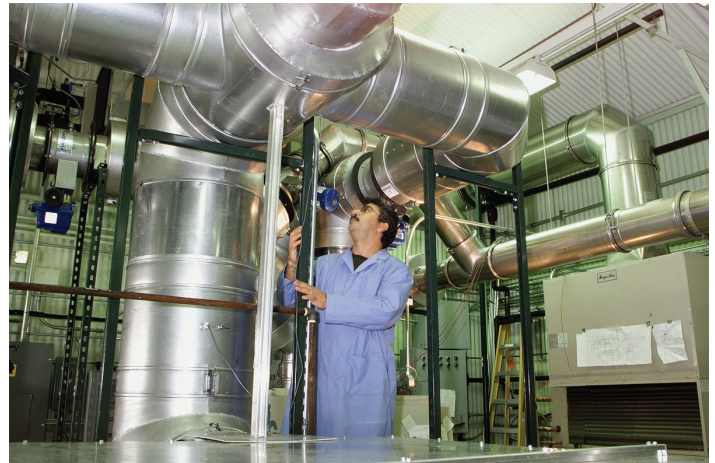
Abdi Zaltash checks equipment inside ORNL's new CHP Integration Laboratory.
