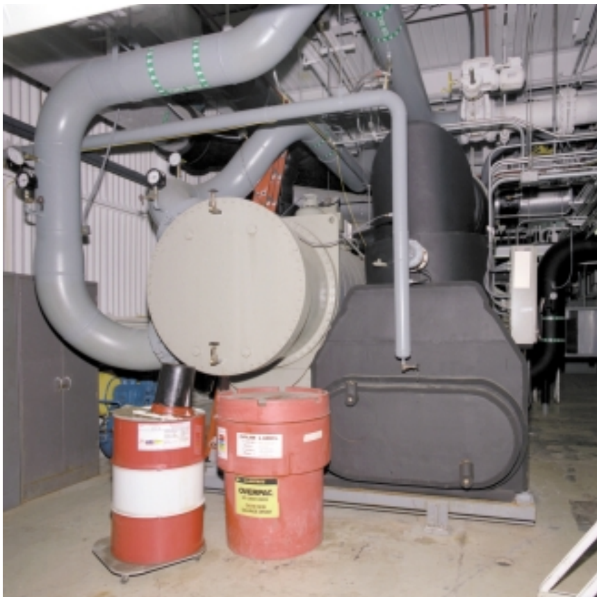
The average steam distribution system, such as this one at ORNL, typically offers savings opportunities on the order of 20%.
