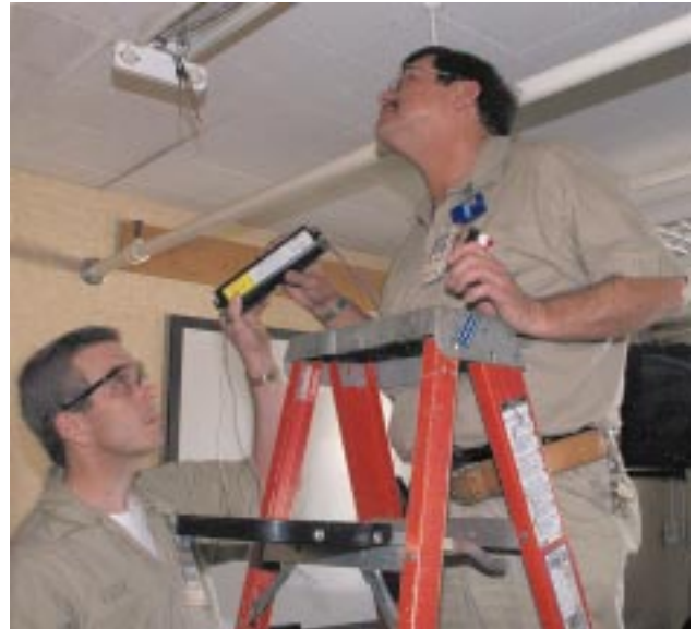
John Price (left) and Gary Ford, electricians at ORNL, replace inefficient magnetic ballasts with energy-efficient, environmentally friendly electronic ballasts.
