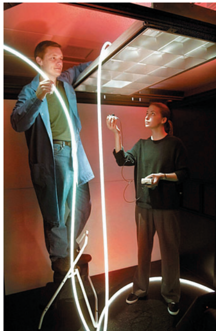
Duncan Earl and Tonya McFadden of ORNL install optical cables in a hybrid luminaire.
