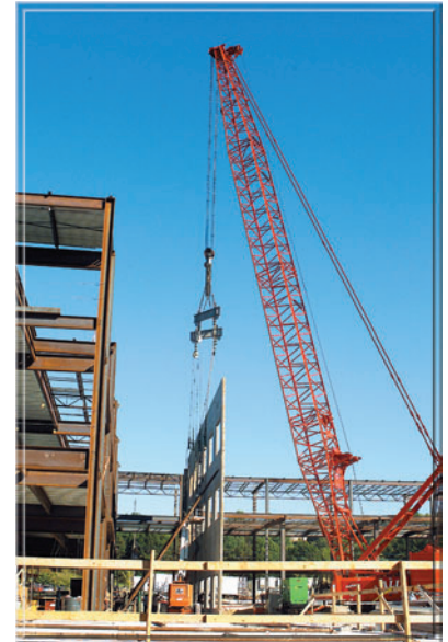
A crane lifts a pre-assembled wall into place on one of ORNL's new buildings.
