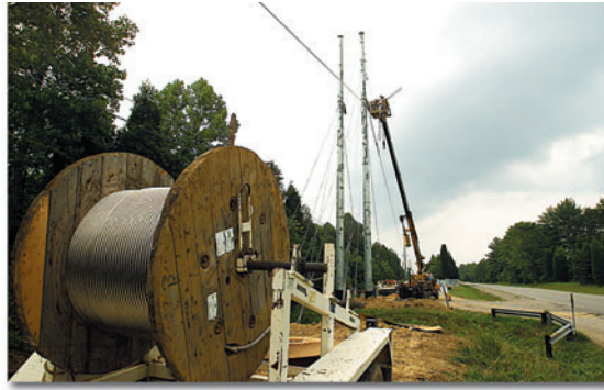
ACCR wires being installed at ORNL's PCAT facility for 3 years of operation and testing.
