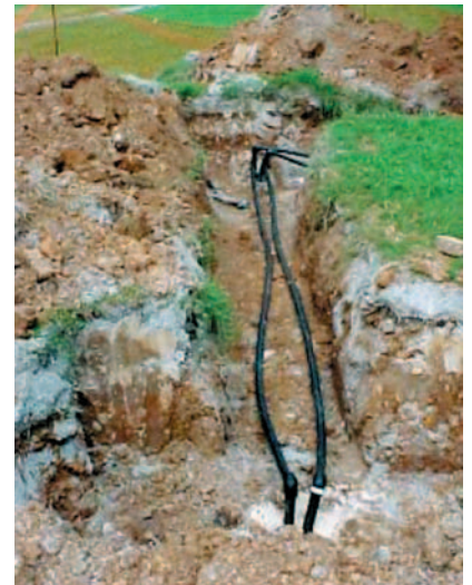
The GHP at the Robertsville school removes heat via a water/glycol solution pumped through these vertical wells bored in the earth just outside the classroom.
