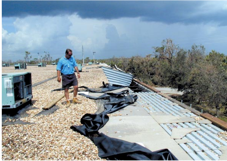
A member of the RICOWI team surveys hurricane damage to the roof of a large commercial building in Florida.
