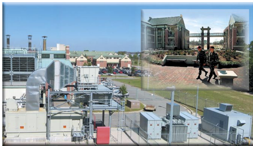
An integrated energy system with turbine generator and absorption chiller provides cooling, heating, and reliable power to barracks at Ft. Bragg.
