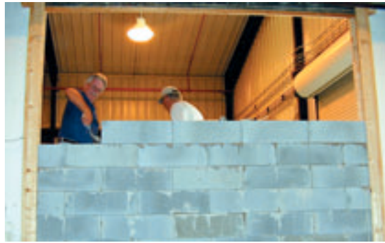
Construction of the flyash test wall in the BTC. The AAC blocks, found to have good insulating properties, will be field-tested in a Habitat for Humanity house.
