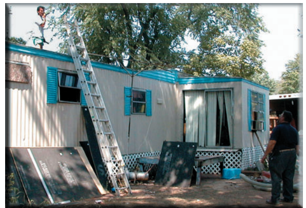
A weatherization crew making energy-efficiency improvements to a mobile home as a result of MHEA Program screening.
