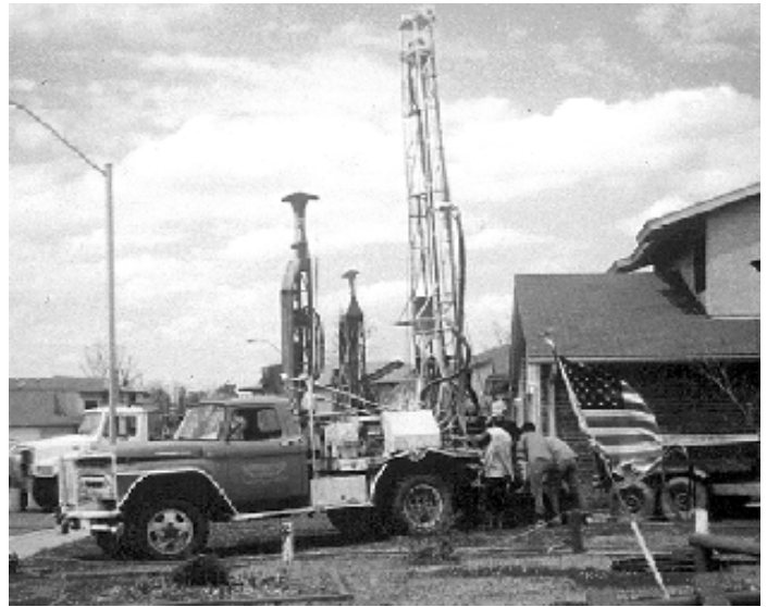
A rig drills boreholes for installation of polyethylene pipe for geothermal heat pump installations at Fort Polk.
