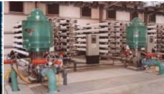
(d) Large RO water purification plant (four each a million gal/d capacity). Courtesy of American Engineering Services Inc.
