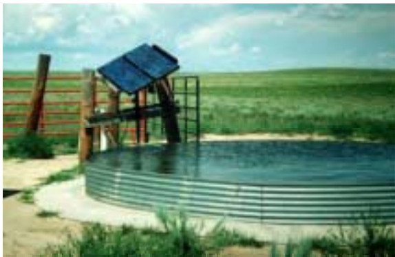
Figure 2.2. A water storage system for cattle watering using a PV pumping system.
