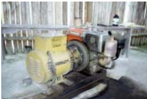
Figure 3.1. Diesel generator at a rural Panamanian hospital.
