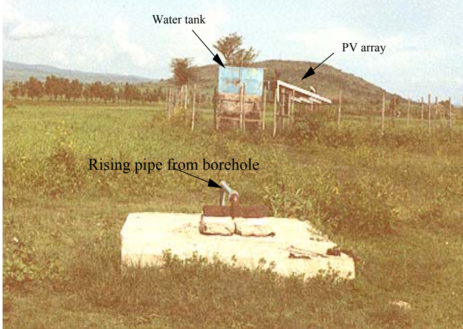
Figure 5-4. A typical village water supply using a PV pump located in Ethiopia. The system has no distribution networks.
