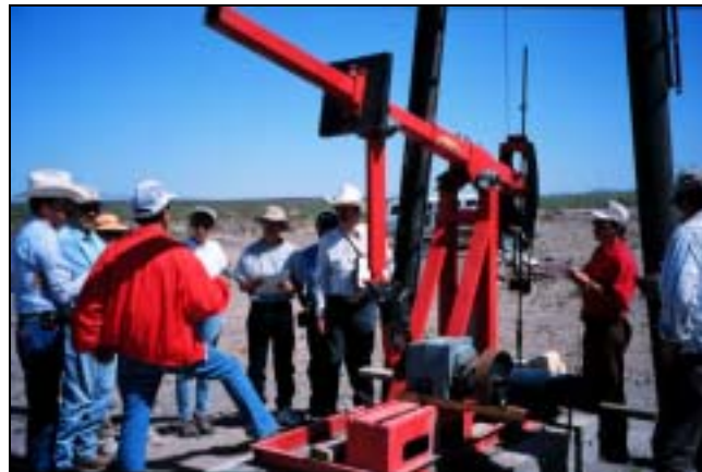
Figure 7-1. Installation of a solar surface pump (jack pump) at Rancho Guadalupe in Chihuahua, Mexico.
