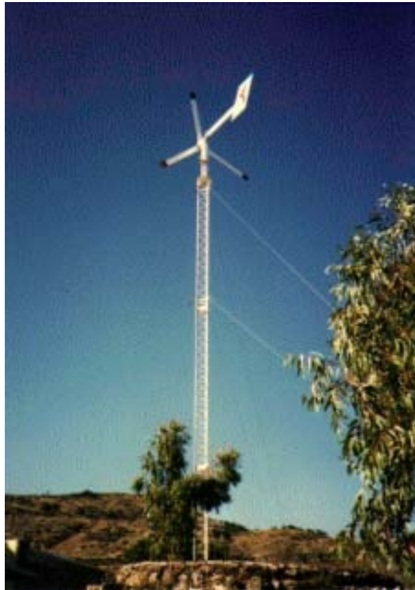
Figure 5-3. A Typical electrical wind pump located at Santa Maria, Mexico.
