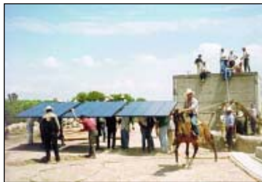
Figure 8-3. Pilot PV water pumping installation in the Mexican State of San Luis Potosí.
