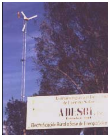
Figure 7-4. Electrical wind water pumping system at the ADESOL training facility near Sosua, Dominican Republic.
