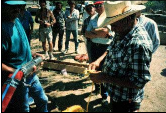
Figure 7-2. Typical submersible pump installation in Sonora, Mexico.
