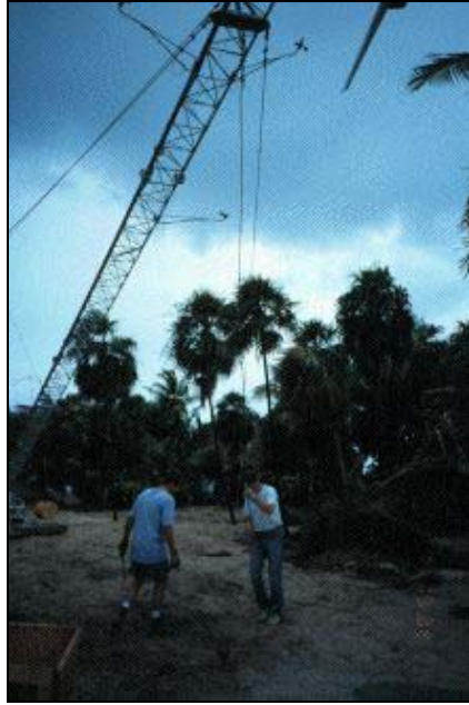
Figure 7-3. Typical tilt-up tower wind system installation (Bergey Excel 10 kW) in Quintana Roo, Mexico.
