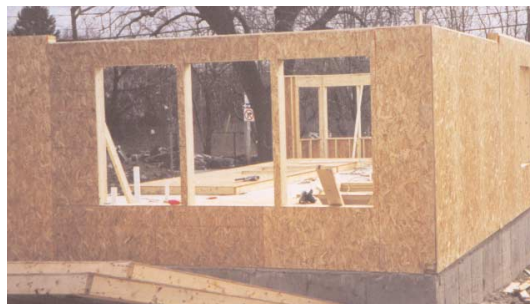
The building frames were assembled off-site in a warehouse, where unused construction materials were recycled, and weather did not affect the construction schedule. As a result, waste and delays were minimal.
