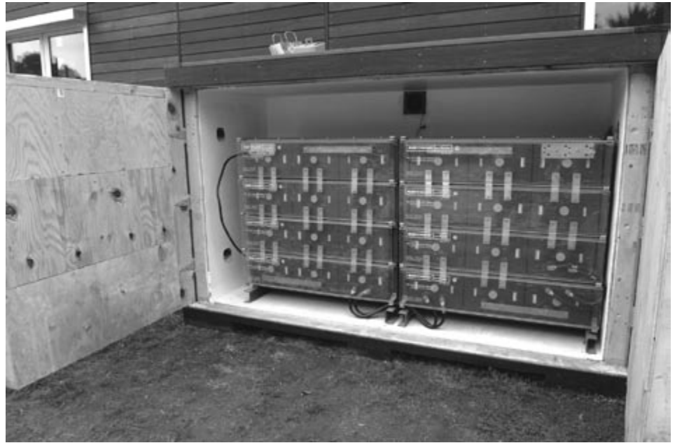
The Cornell team's ingenuity shows with their use of under-the-deck space for battery storage, which obviates the need for a separate space inside the house. A rule change for the 2007 Solar Decathlon allows battery storage outside the footprint of the house.
