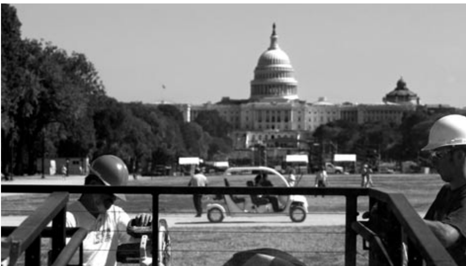
On October 5, when this picture was taken, the 2005 Solar Decathlon opening ceremony was just a day away and the solar village hummed with activity. Pictured are members of the Cal Poly team installing safety wires on their ADA-compliant ramp.
