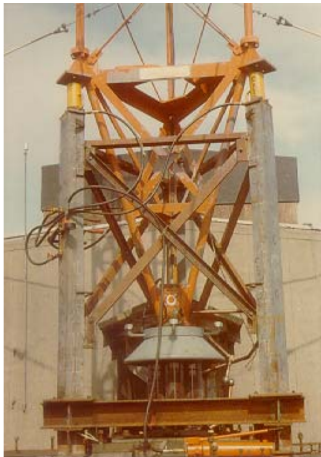
Figure D-4 Jacking Frame utilizing jack at the upper end. Note restraining guys that are visible at the top of the photo.
