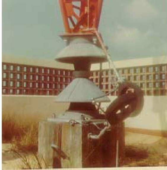
Figure 5-4 Double cone base insulator.
