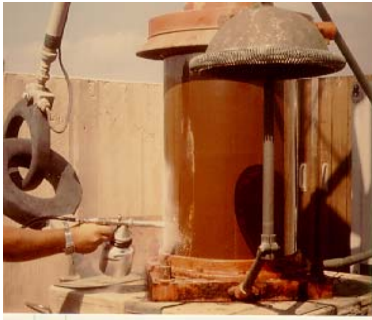
Figure 5-7 Statifluxing an oil-filled base insulator.
