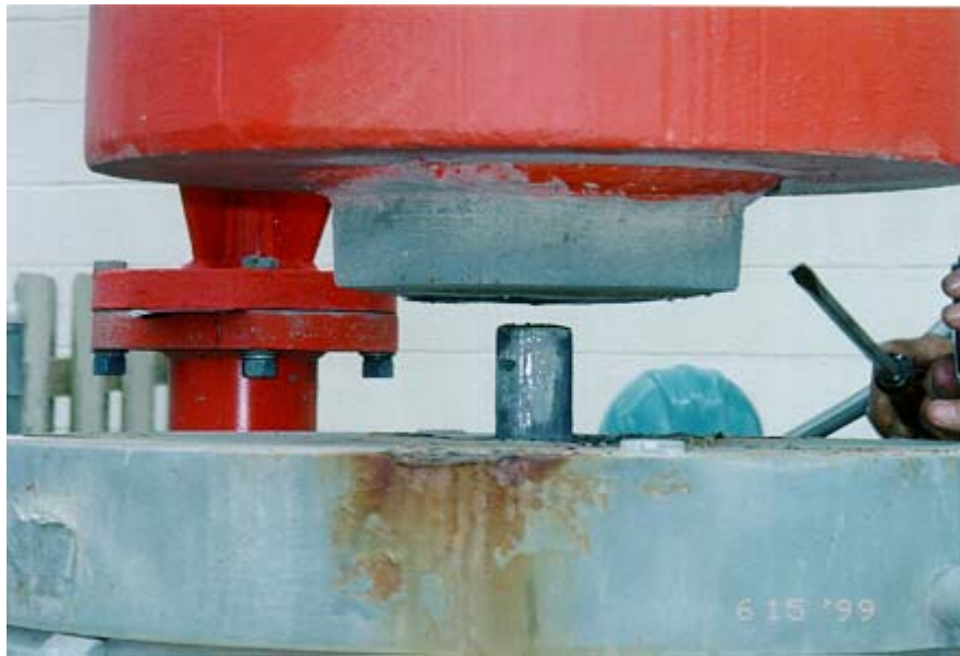
Figure D-9 Tower jacked up to approximately 1/2-inch above center pin of base insulator.
