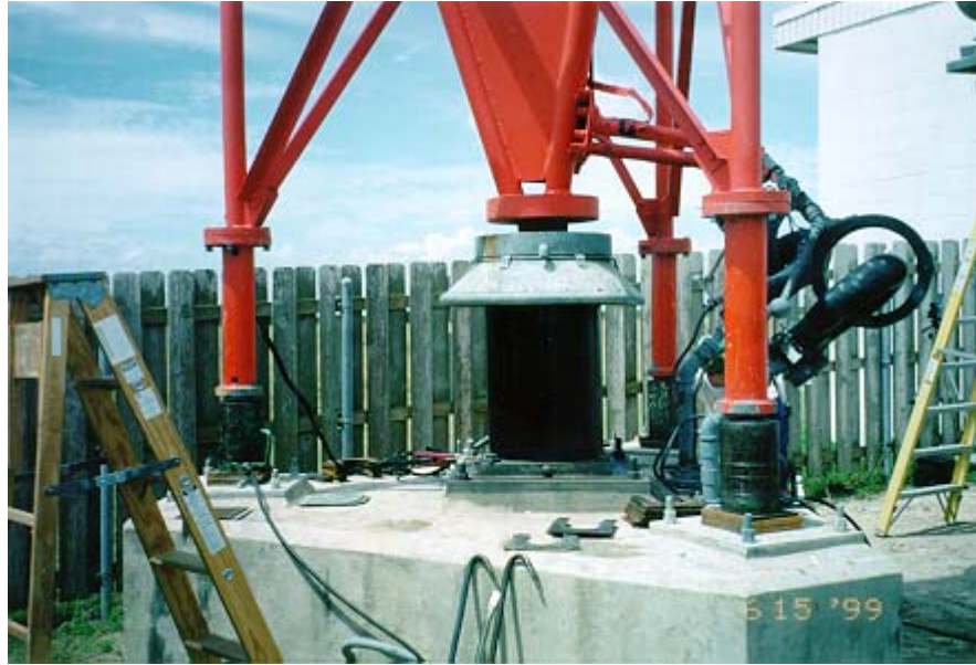
Figure D-1 Tower jacking legs installed on permanent jacking frame prior to insulator replacement.
