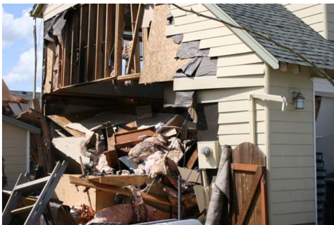
View of the destroyed garage side wall and second floor debris after the explosion
