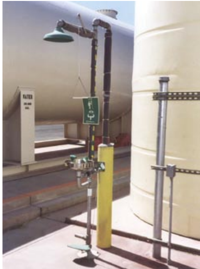
Figure 64—Emergency eyewash station (San Bernardino, CA).
