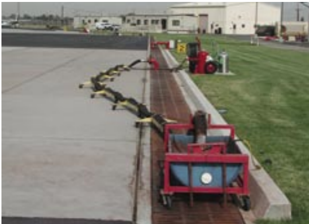
Figure 30—Loading pad wash down water collection trench with grating (San Bernardino, CA).
