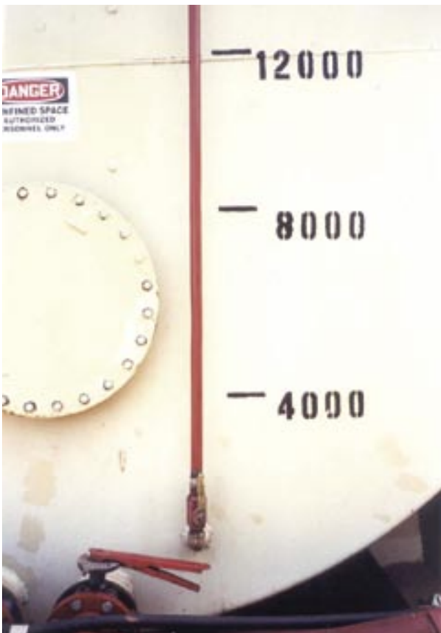
Figure 51—Tank liquid level sight gauge.
