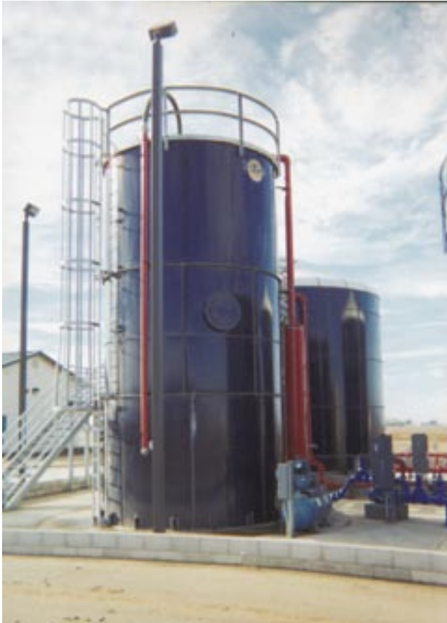
Figure 17—Dry powder retardant storage silo (Porterville, CA).
