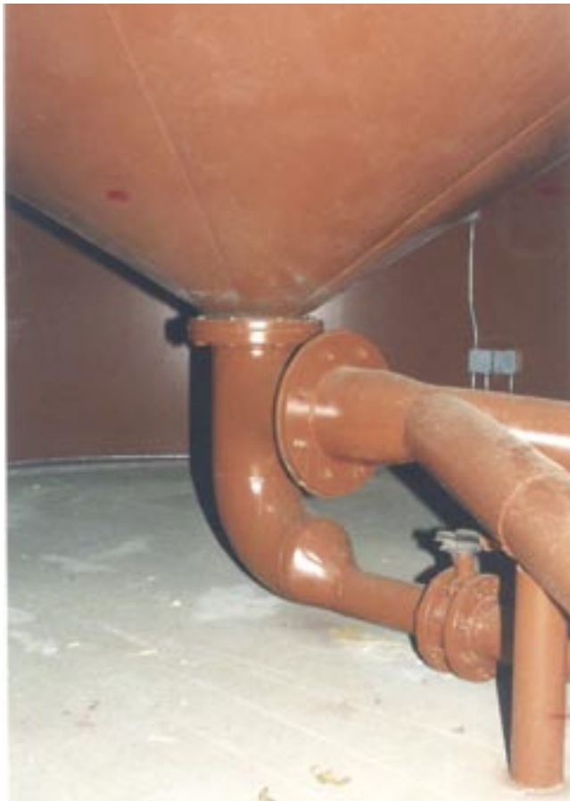
Figure 50—Conical bottom storage tank with debris trap installed at tank outlet.
