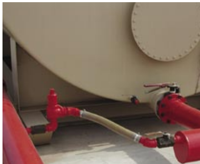
Figure 59—Pressure relief valve (San Bernardino, CA).
