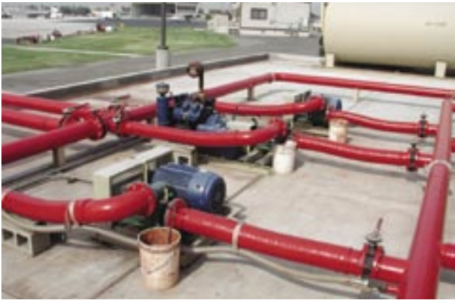
Figure 48—Electric- and gasoline-powered retardant pumps with vibration isolating flexible hose (San Bernardino, CA).
