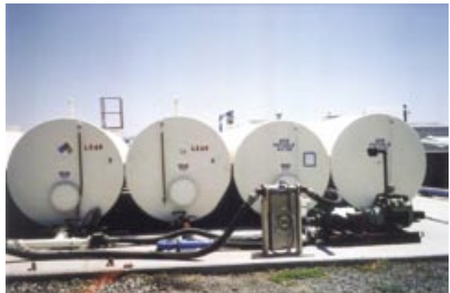
Figure 42—Wet-concentrate storage tanks in a spill-containment pit (Stead, NV).
