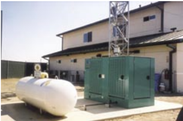
Figure 73—Retardant base backup electric generator system (Porterville, CA).
