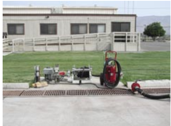
Figure 32—Loading pad utilities (San Bernardino, CA).
