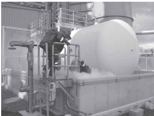
Ammonia tank leak
