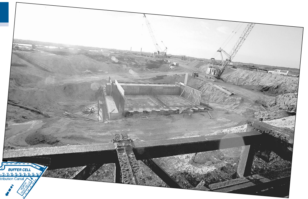
The construction of flow-through treatment marshes, known as Stormwater Treatment Areas, in Loxahatchee National Wildlife Refuge will remove excess nutrients from agricultural runoff to help restore the Everglades ecosystem.
