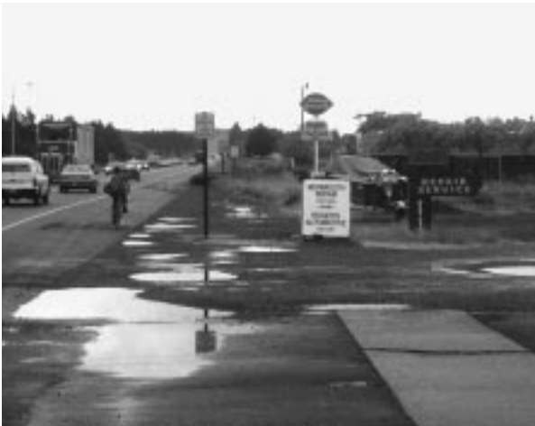
Sidewalk ends abruptly
