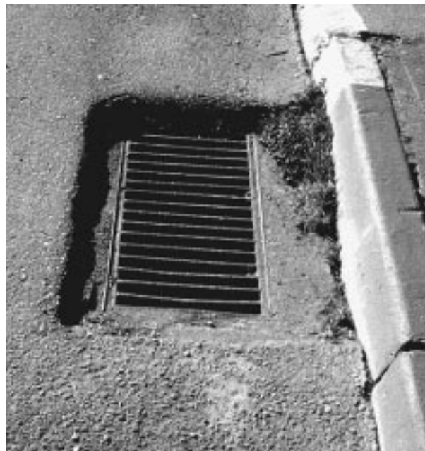
This catch basin should have been raised after pavement overlay
