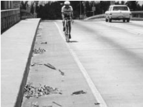
Debris accumulated on the shoulder forces cyclist into the roadway
