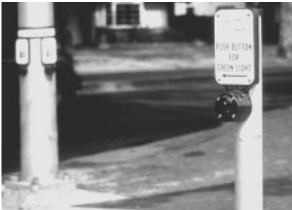
Push-buttons on poles and pedestal
