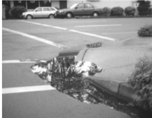
Poor drainage traps water in crosswalk
