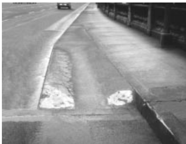
This ramp allows bicyclists to ride straight onto bridge sidewalk
