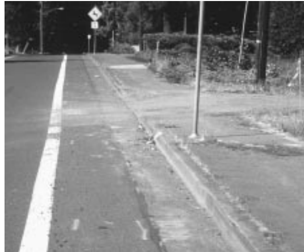
Construction operation leaves debris in bike lane
