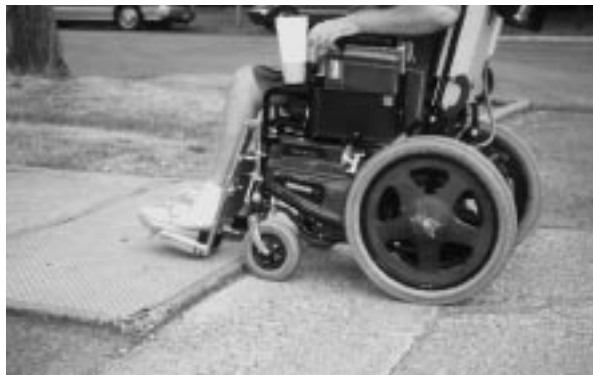
Wheelchair can't proceed here
