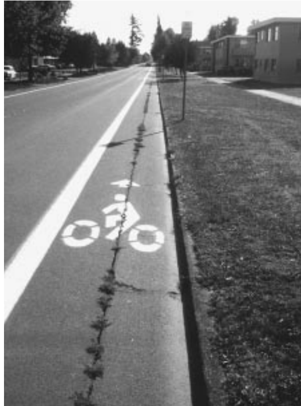
Weeds breaking up bike lane
