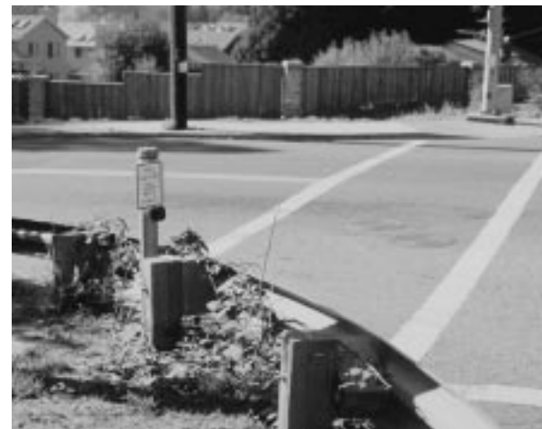
Crosswalk is inaccessible because of guardrail
