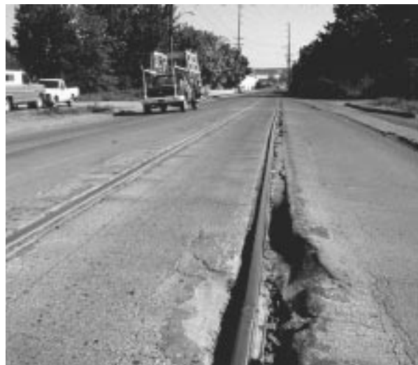
Extremely undesirable condition
