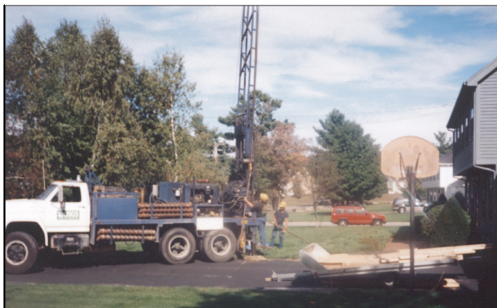
Drilling a shallow well in an urban area in the Boston metropolitan study area.
