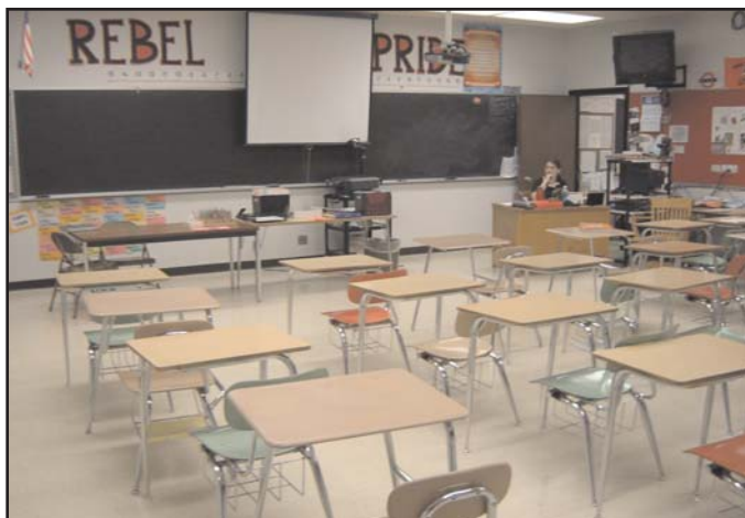
Students and teachers can enjoy new lighting fixtures that use less energy thanks to the measures installed under the ESPC.
