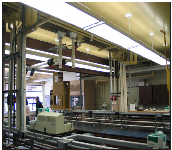
The labs at the Hatfield Marine Science Center have updated lighting, new controls and safer heating equipment.
